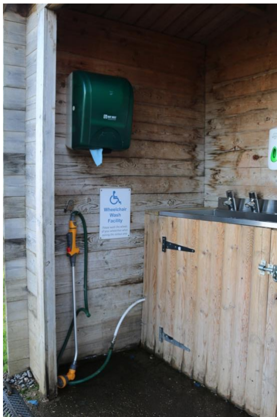
Wheelchair wash station
